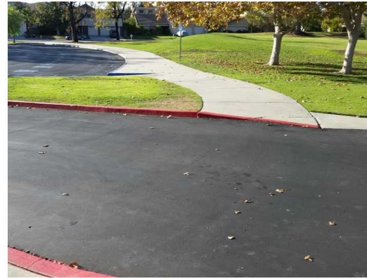
Photo 1 The accessible path from the ADA parking stalls to the Administration is not continuous.
